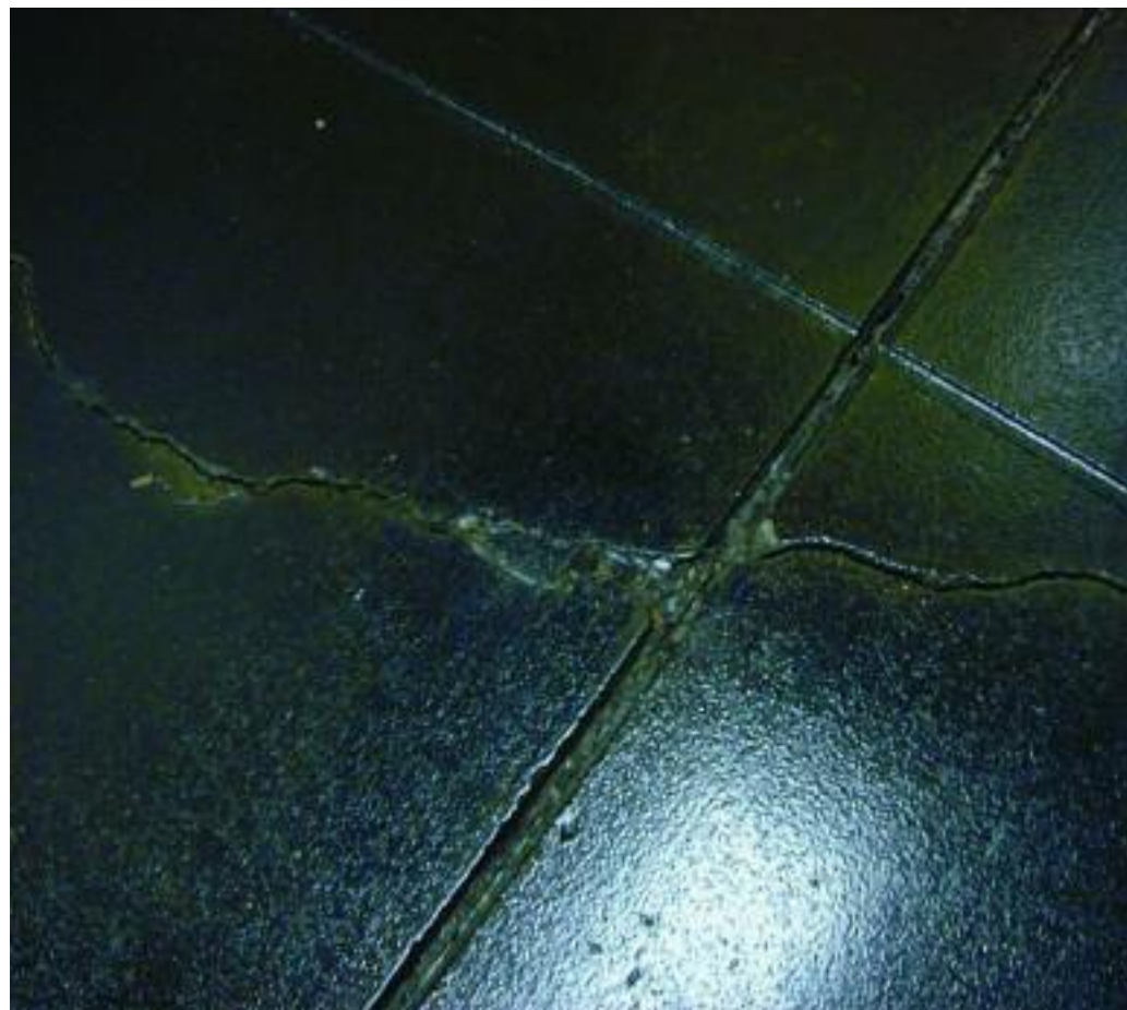
Right: Cracked tile may be due to shrinkage of a concrete subfloor or deflection in a wood subfloor.
